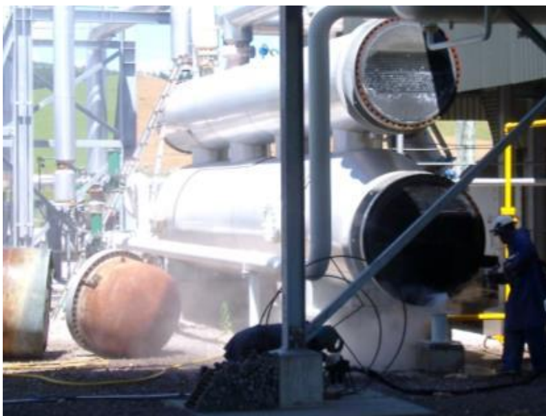
Figure 3.18 : Binary plant heat exchangers (large plant example)
