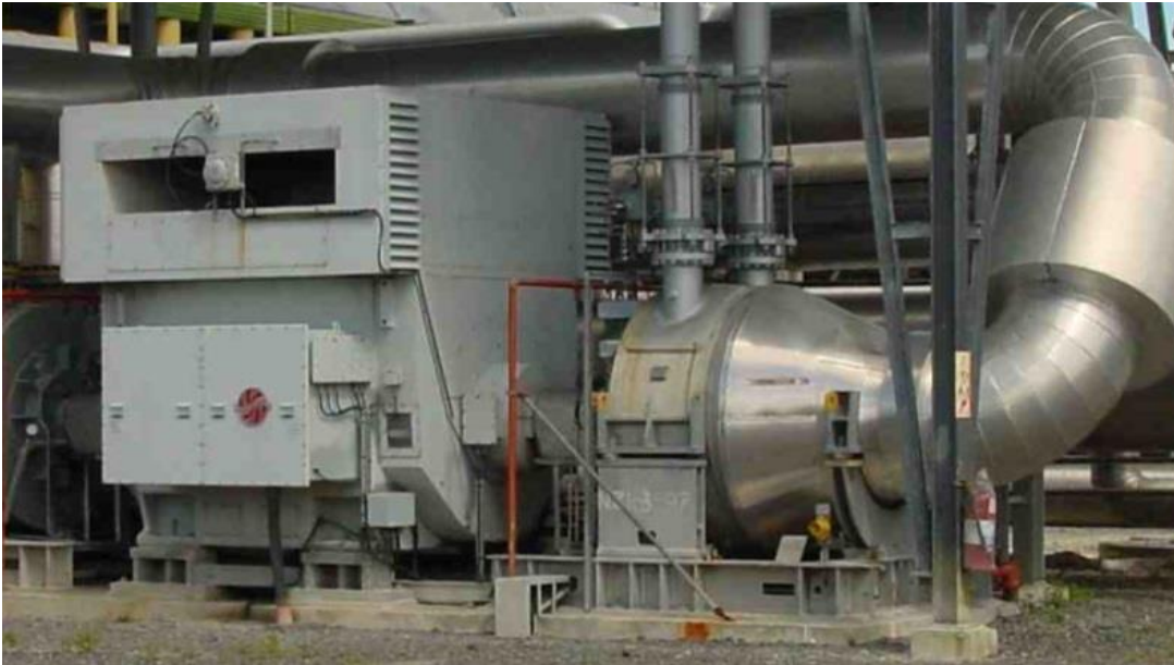
Figure 3.20 : Typical 5.8 MW generator (Ngawha Power Station, New Zealand)
