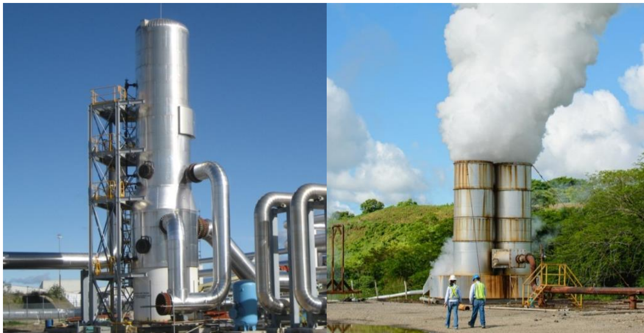
Figure 3.11 : Typical geothermal separator and Atmospheric Flash Tank (AFT / Silencer)
