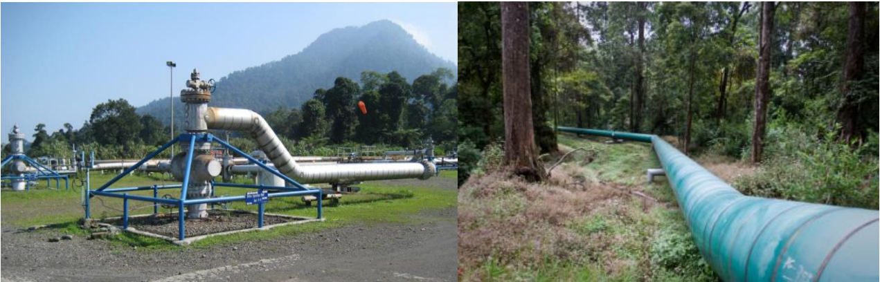
Figure 1.6 : Typical Production Well (left) and Reinjection Pipeline (right)
