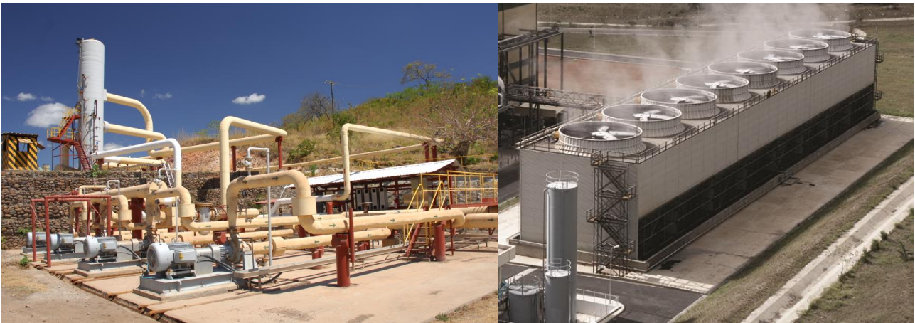
Figure 1.7 : Typical Bringe Pump (left) and Cooling Tower only 1-2 cells likely required for Dominica Project (right)
