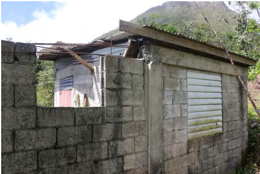
Figure A-4: Residential Structure Incomplete C3
